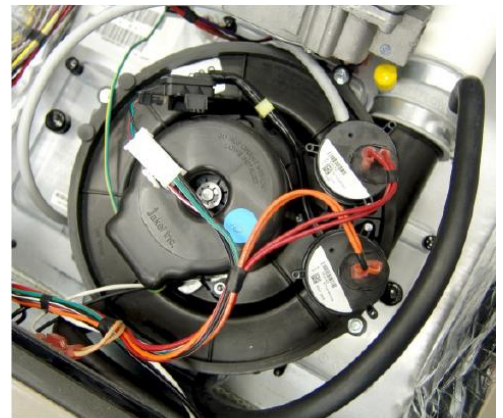
Induced Draft Blower
