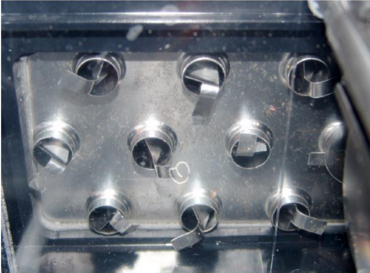
Outlet of the Secondary Heat Exchanger, with the Turbulator Strips Visible
