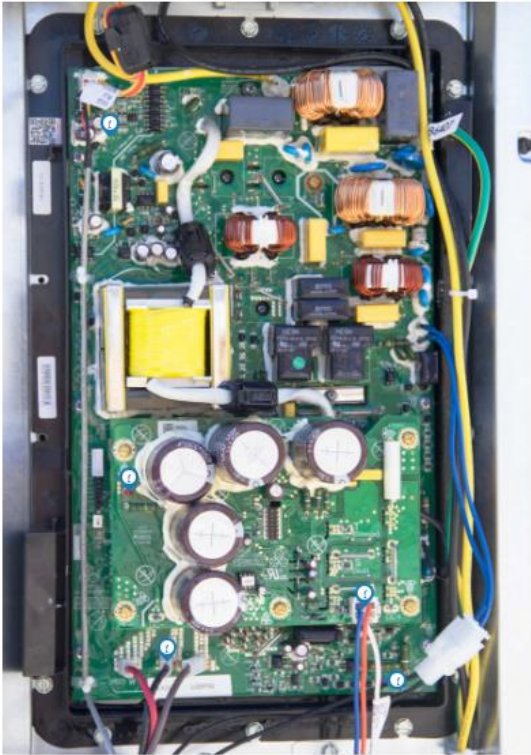
Inverter (Cover Removed)
