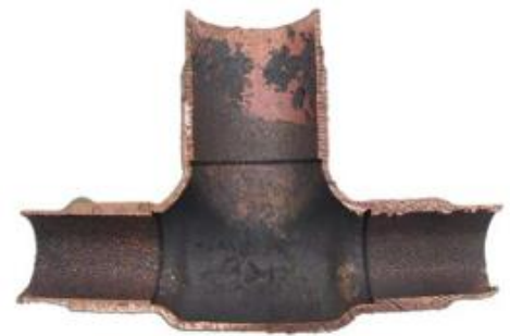
Oxidation Caused by Brazing Without Nitrogen Purge
