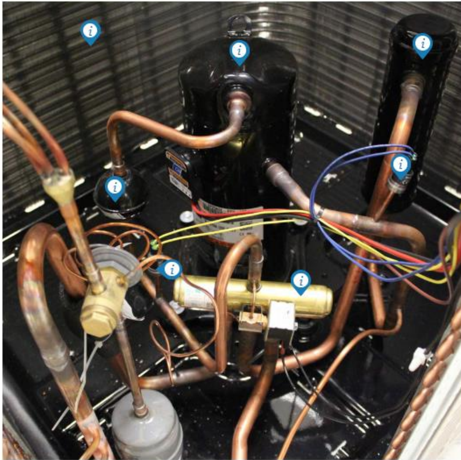
Heat Pump Interior
