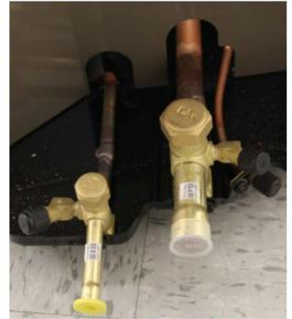
Liquid Line & Suction Line Service Valves
