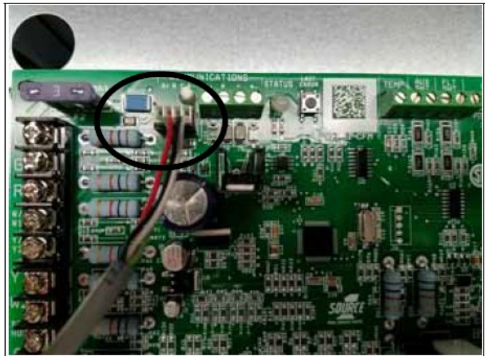
FIGURE 30: Communicating Port of the Furnace
