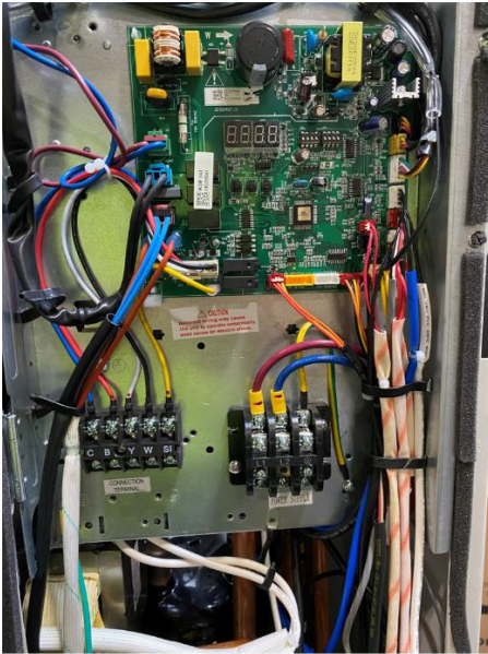
The control board for the HMM7-4 and 5 ton
