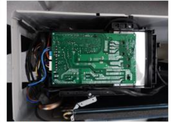
Main Control Board (Under Top Panel)
