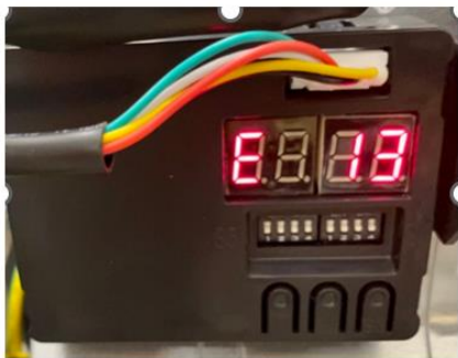
Example of a Outdoor Fault Code #13 Compressor Overheat Protector Device
