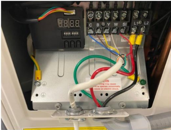
Incoming Wiring: Low Voltage and Line Voltage
