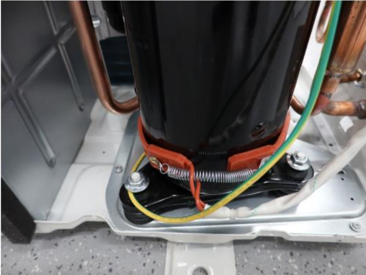
Compressor Heating Belt (Crankcase Heater)
