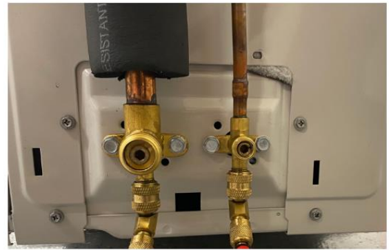
Refrigerant Access Valves (Caps Removed)
