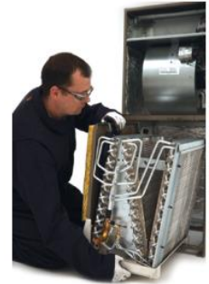
Air Handler Coil
