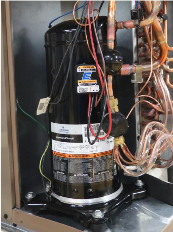
Two Stage Compressor
